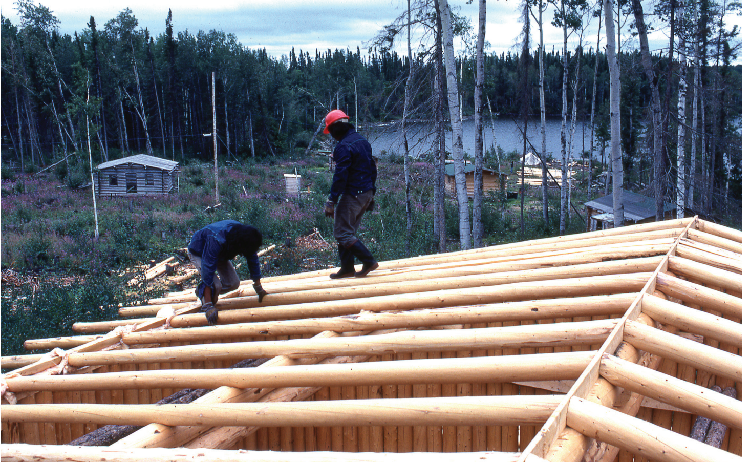
Image 1: Two community members work on the roof a house in what is now Old Town (Courtesy of Tommy Yellowhead).
